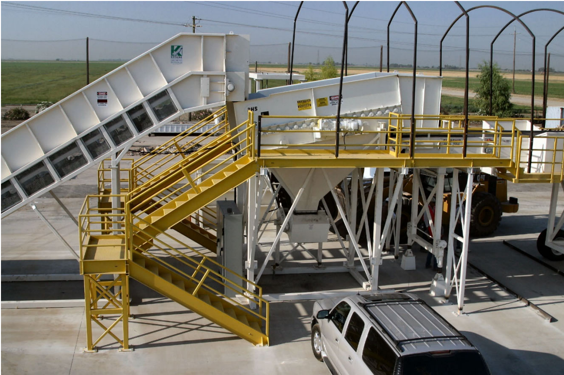
Figure 1: Incline infeed conveyor and mechanical screen for proposed C&D Processing Line
