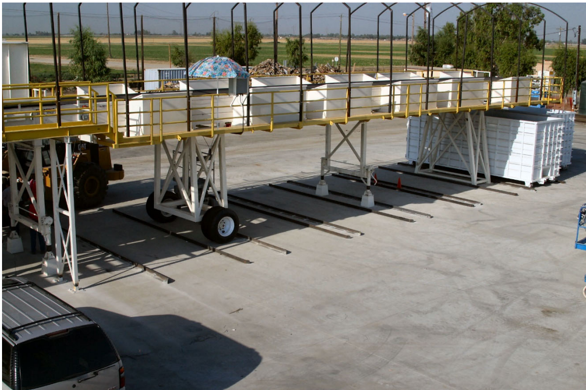
Figure 2: Sorting platform and takeaway conveyor for C&D Processing Line
