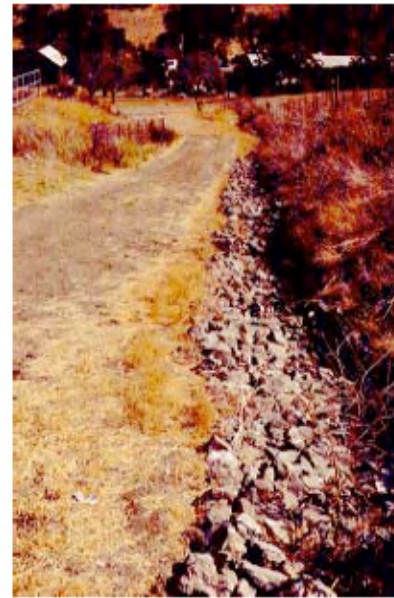
A rock-lined ditch is necessary along this steep road. Well-constructed and maintained ditches are key to the long-term stability of an insloped or a crowned road.
